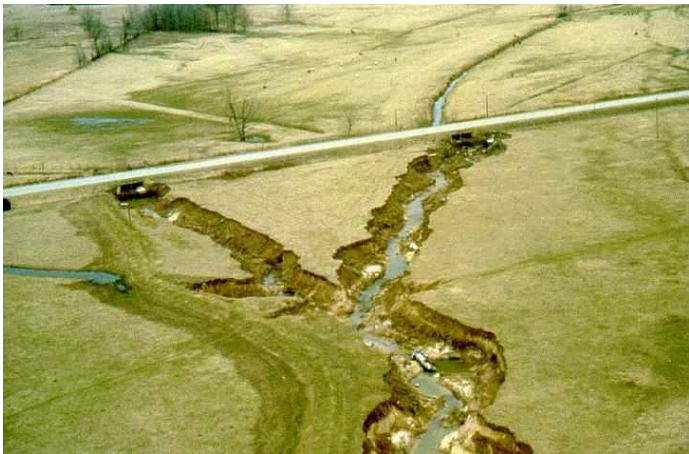
Headcuts and bank failures worked their way upstream (photo by US Army Corps of Engineers).
