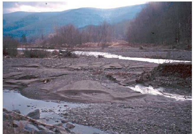
This stream segment was over-widened with bulldozers to make room for floodwater (photo by NY City Department of Environmental Protection).
